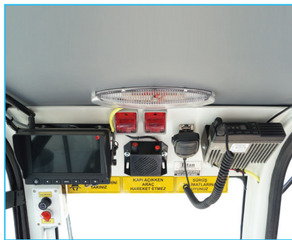
Intercom between personnel and operator cabin, Personnel door open indicator in the operator cabin
